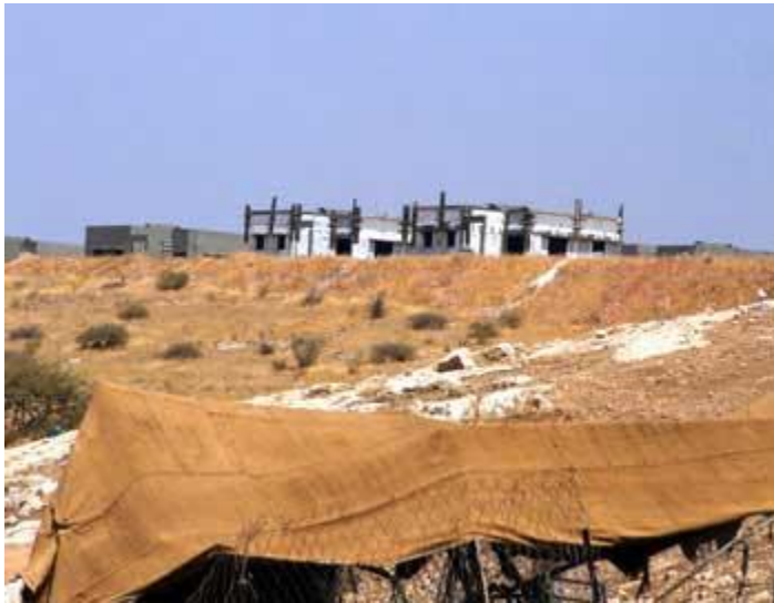
New construction in the Maskiyot settlement, which was built next to 'Ein al-Hilweh. Residents of the settlement were given a permit to continue the construction during the building freeze in the settlements. Photo: 'Atef Abu a-Rub, B'Tselem, 10 August 2010.
