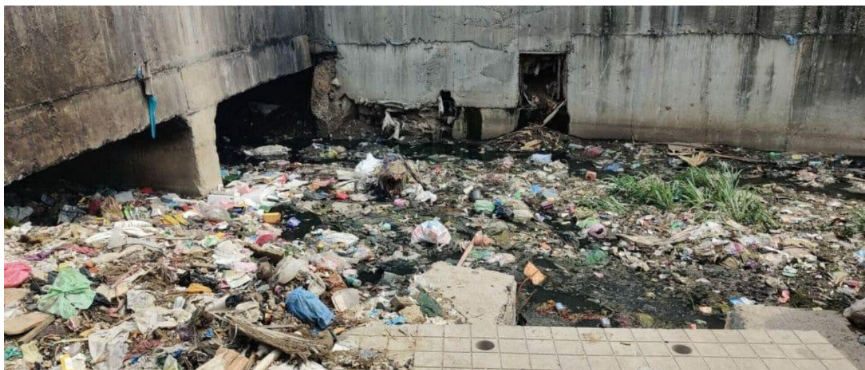
Figure 13: The stormwater drain at Ejipura, filled with garbage. Source: Pinky Chandran.
